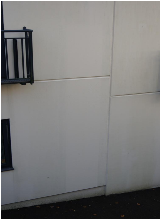
Test area after 5 months. We can now see very clearly where Pureti Clear is applied. The test area is completely clean while the surrounding area has absorbed color from acid rain and greenery.
